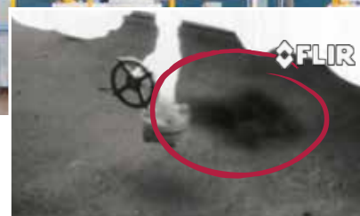
Captured gas leak from production site.
