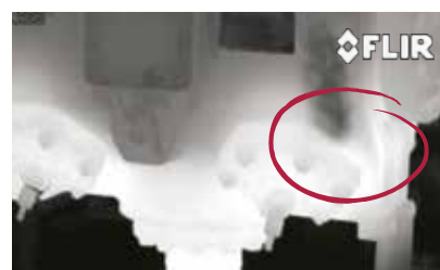
Captured gas leak.
