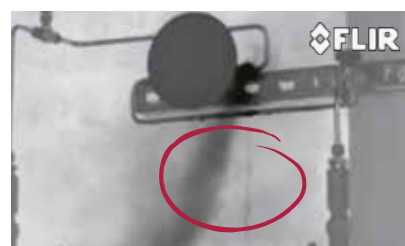
A leaking pressure gauge.
